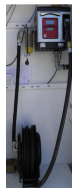
QEII Bulk Tank – TK02
