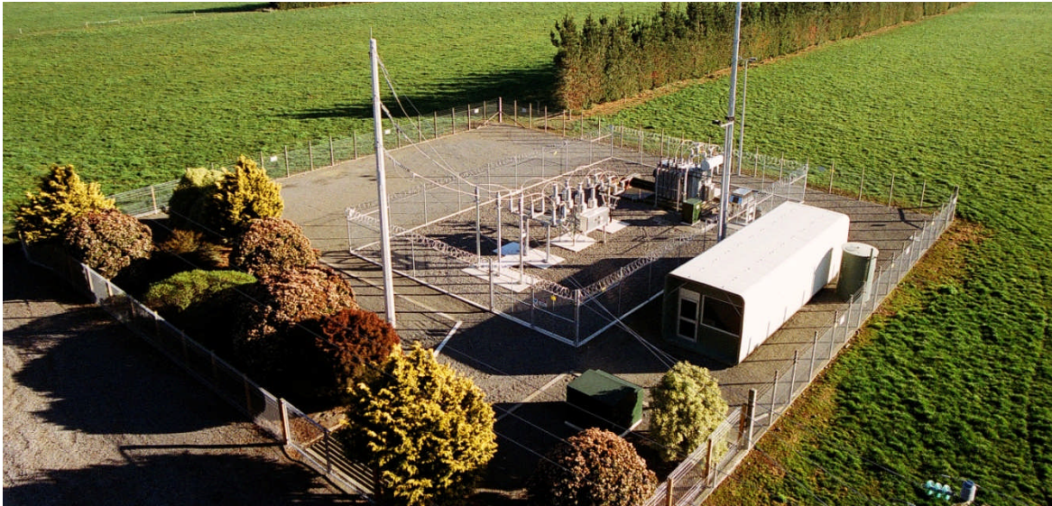
Figure 4: Bankside 33/11kV Zone Substation
