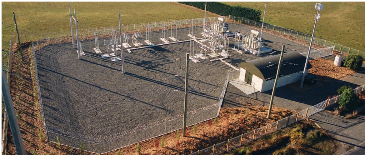
Figure 3: Weedons 66/11kV Zone Substation
