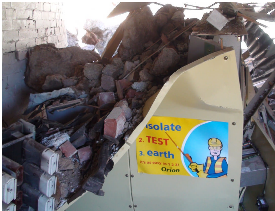
Figure 19: Wakefield Avenue North Substation
