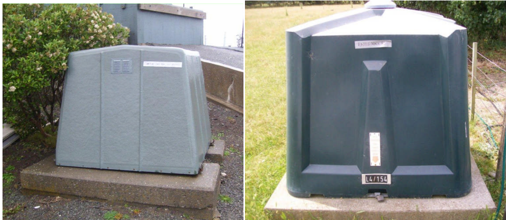
Figure 18: Example of Fibreglass and Polythene Transformer Covers
