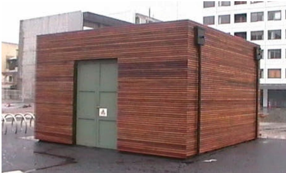
Figure 8: Example of Reconditioned Re-clad Network Substation – Liverpool CFM Sub
