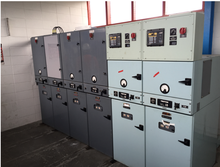
Trentham substation indoor switchboard
