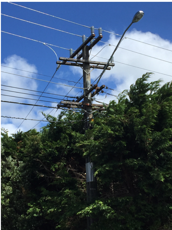
Example of vegetation encroachment on overhead line
