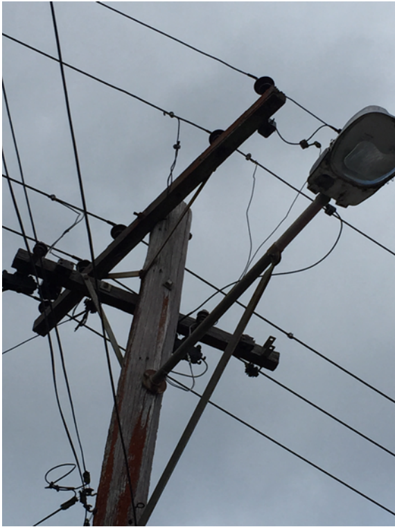
Same LV wood pole showing split in crossarm, loose LV insulator and decay at pole top (not visible on photo)
