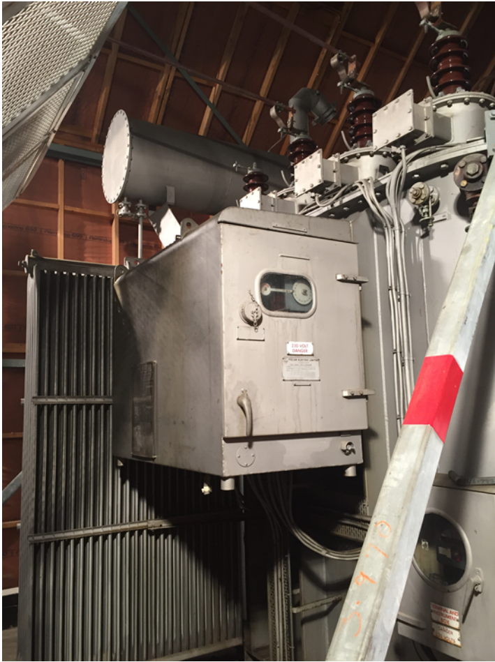
33/11kV substation transformers within new enclosure, which appear in good condition for their age.
