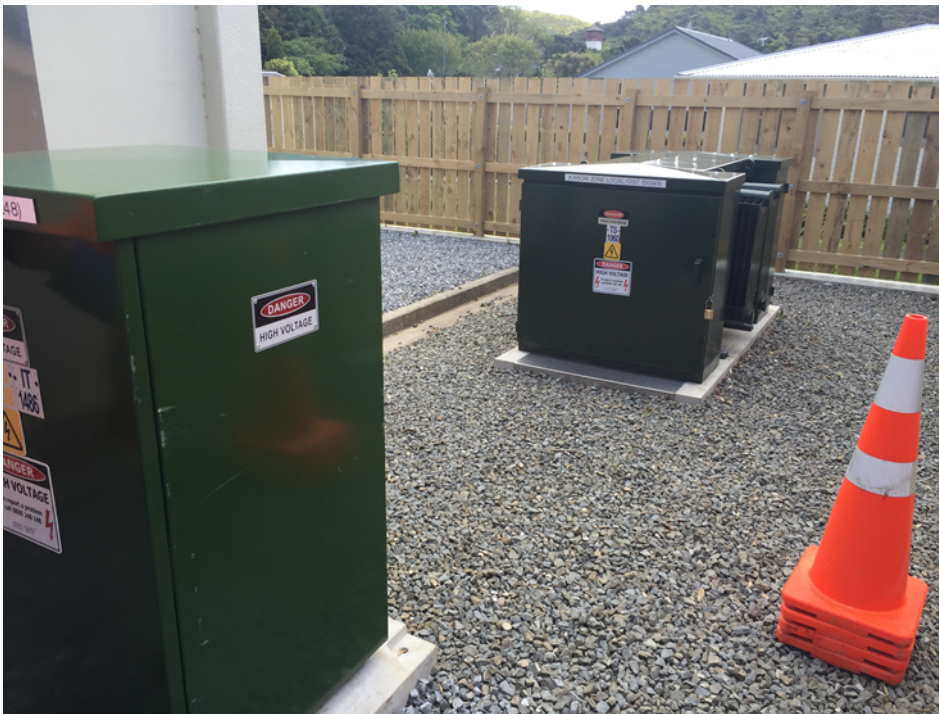
New ground mount distribution substation at Karori substation, separate distribution transformer and switchgear
