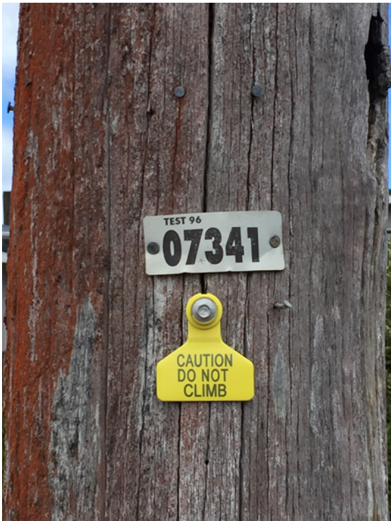
Same LV pole showing non-regulatory yellow tag following inspection. Pole strength ok, however pole decay at top and requirement for new crossarm is likely to be more efficient to replace pole. Timeframe 12 months
