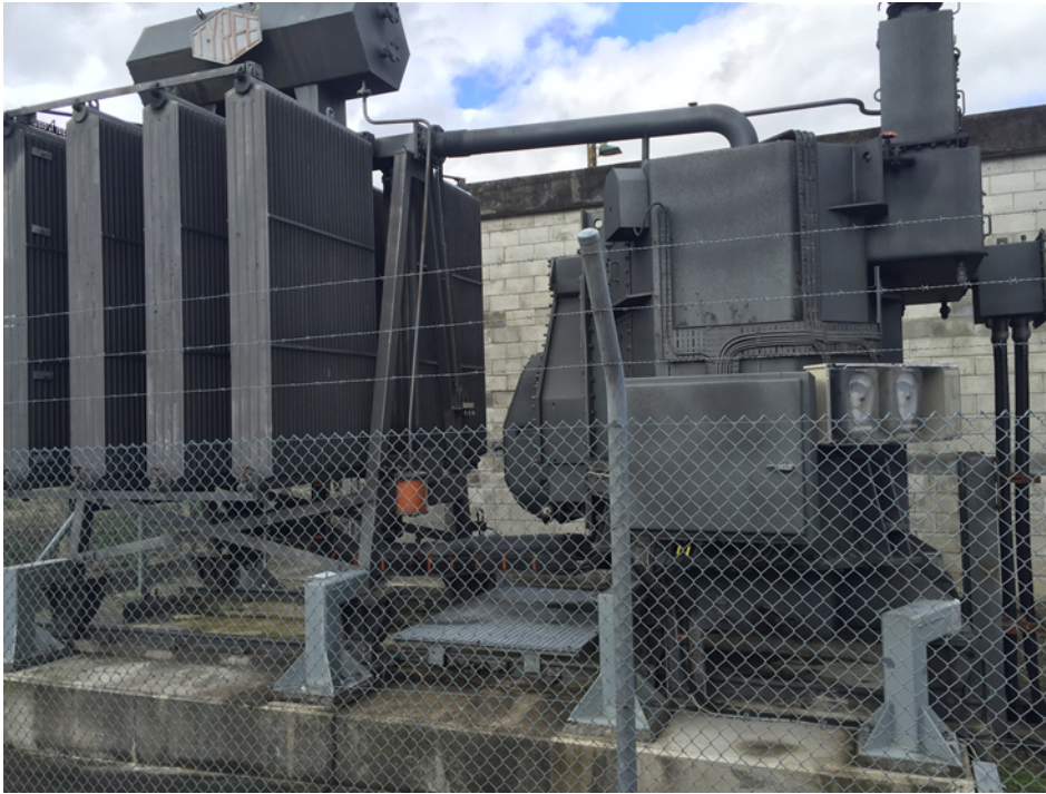
Trentham 33/11kV transformer showing addition of seismic strengthening
