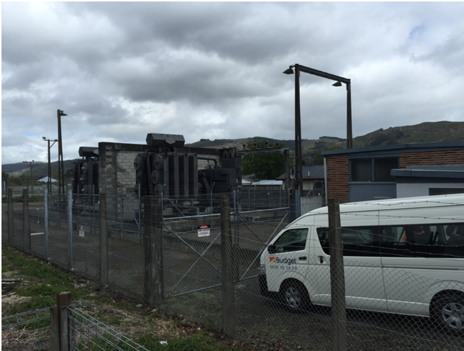
Trentham substation showing switchroom, outdoor transformers and fencing
