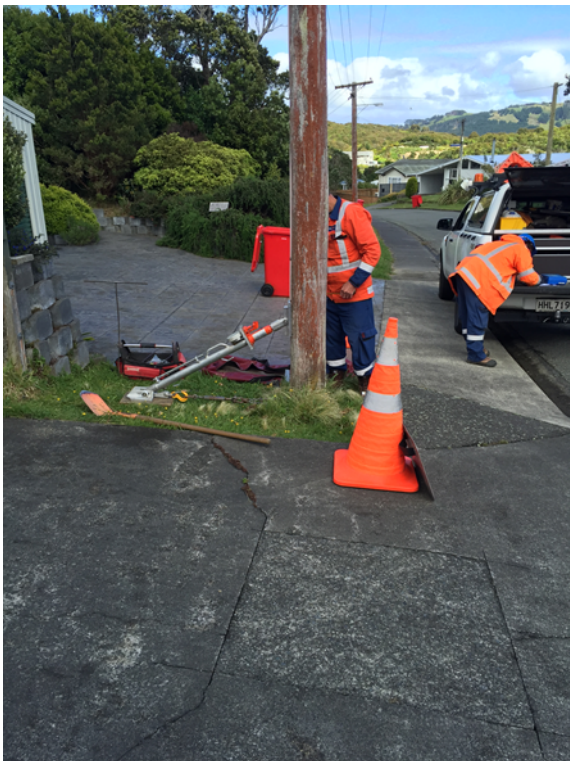
LV wood pole – dueur pole test, Western Hills area
