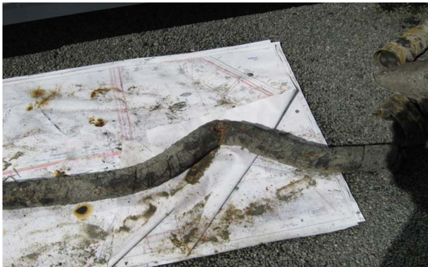
11kV cables were similarly damaged
