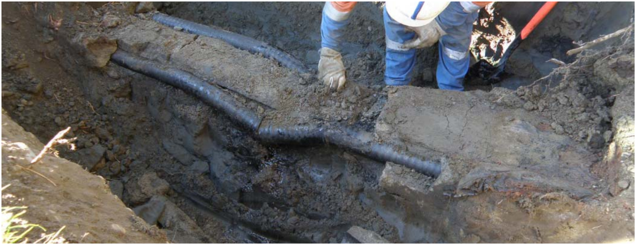
66kV underground cables stretched and broke through ground movement
