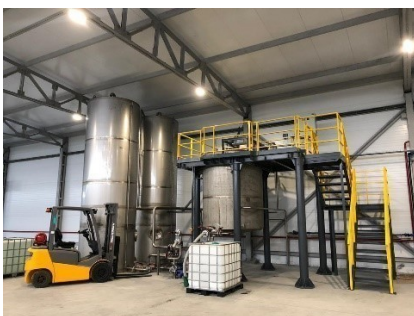
Admixture production plant
