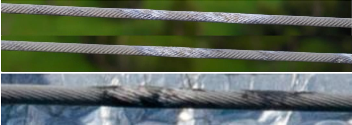
Figure 5: Examples of conductor defects showing corrosion bulging (span T78 – T79 and T129 – T130)
