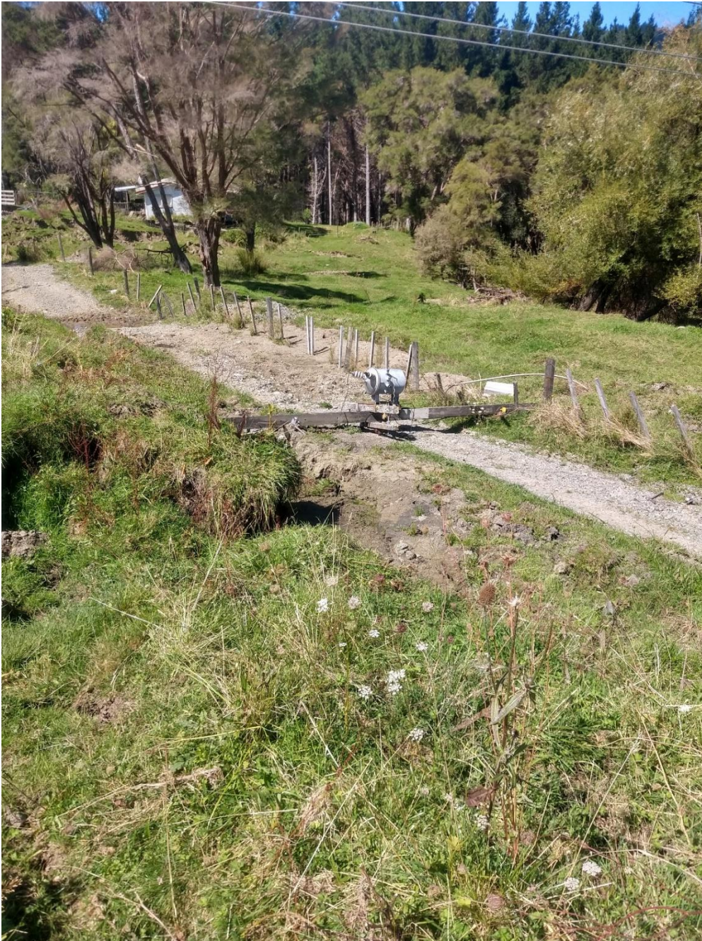
Large landslide North of Tokomaru Bay cause pole to fall over.
