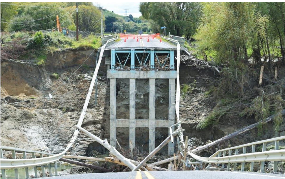
Bridges, water pipes and sewage systems were wiped out by the force of the hurricane when it hit Tairawhiti last year.
