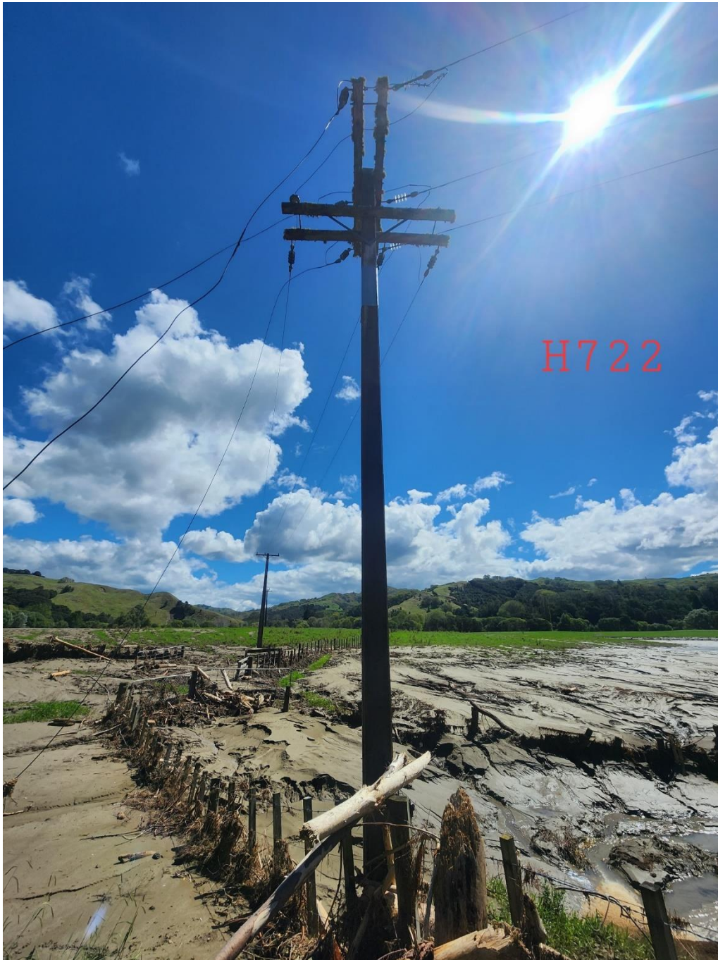
Waiapu road by Waiapu road - wires down due to flooding, slips and tree through line
