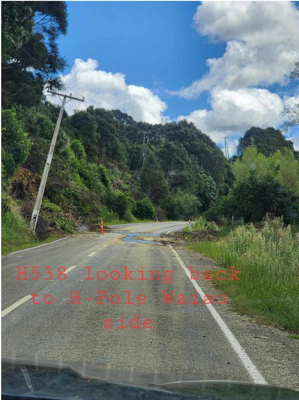
Waiapu Road - tree through lines after flooding and slips
