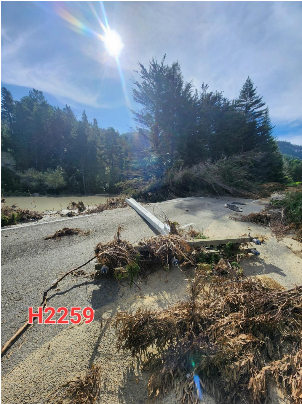
Mangahauini Gorge - Major flooding, landslides causing trees fall through the lines
