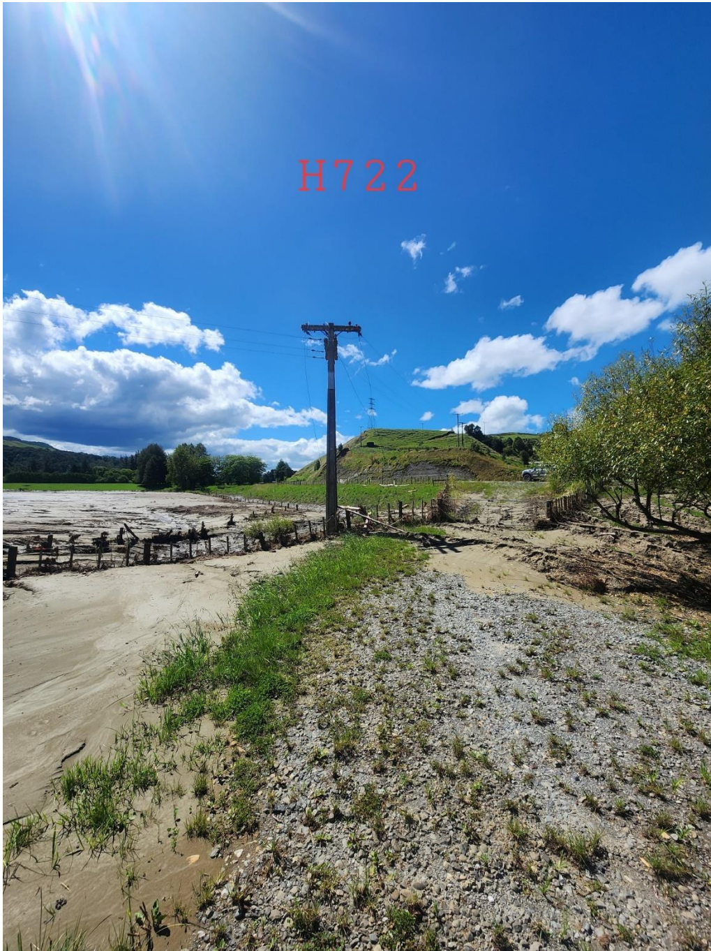
Waiapu Road - flooding and slips
