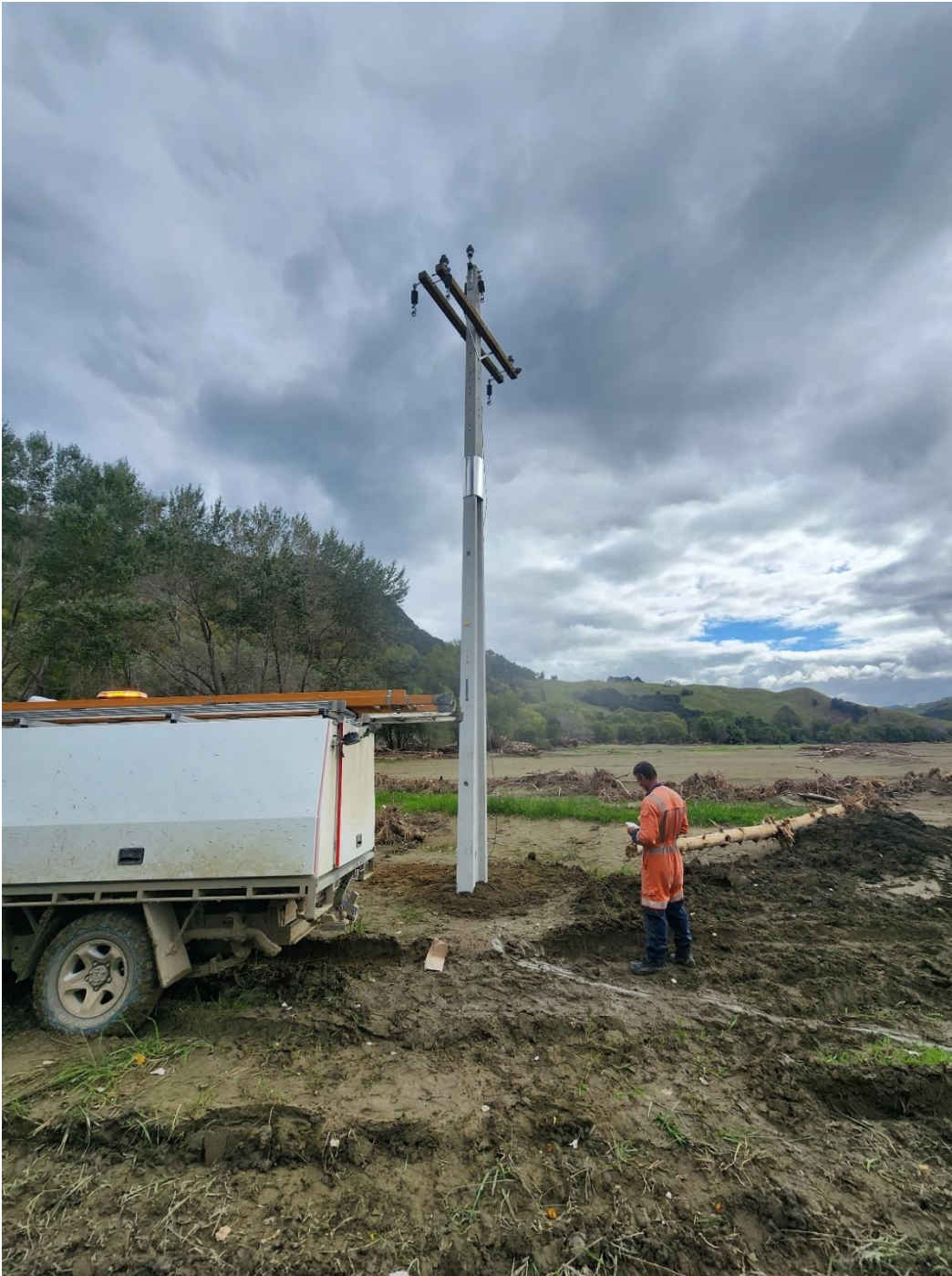
New pole installed to replace pole (H714) washed away at Waiapu road
