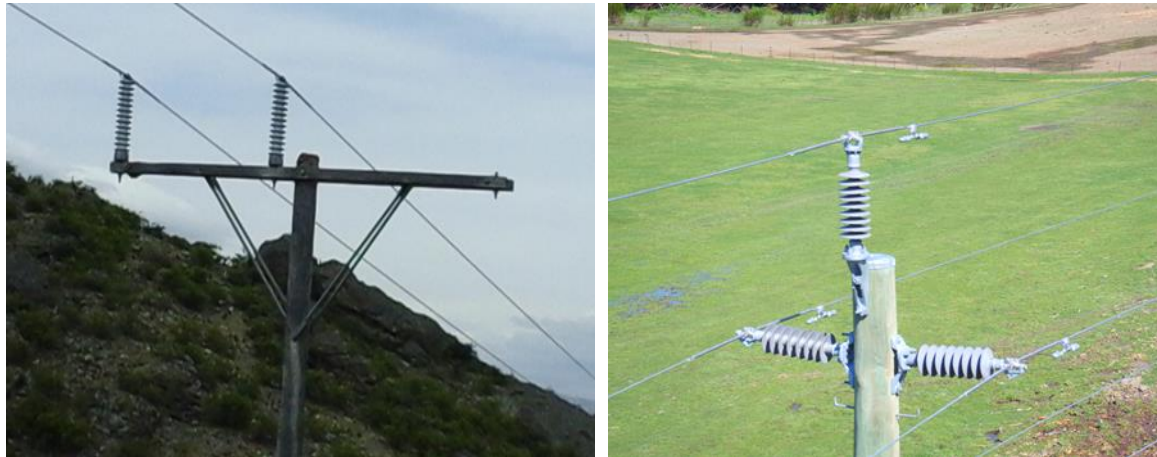
Figure 8.19: Floating conductor following insulator failure (left), and lightweight polymer insulators (right) 72
