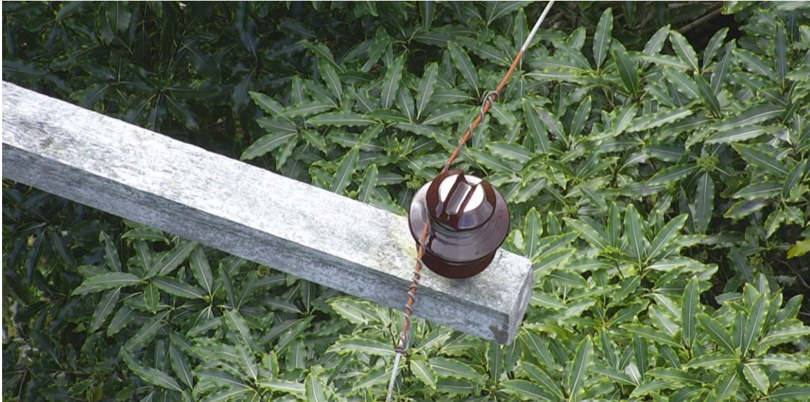
Figure 8.25: Rusted No. 8 wire at an insulator tie point due to bimetallic corrosion with copper tie
