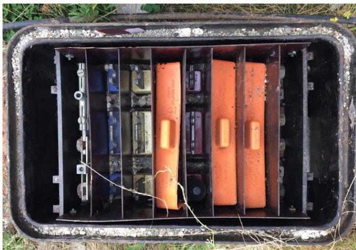
Figure 8.78: Decommissioned Henley underground link box
