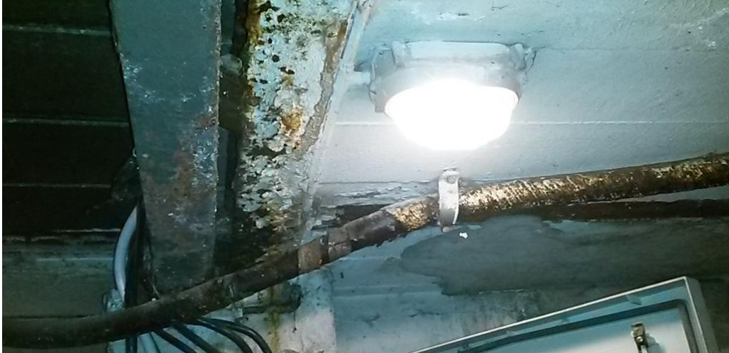
Figure 8.83: Example underground distribution substation condition
