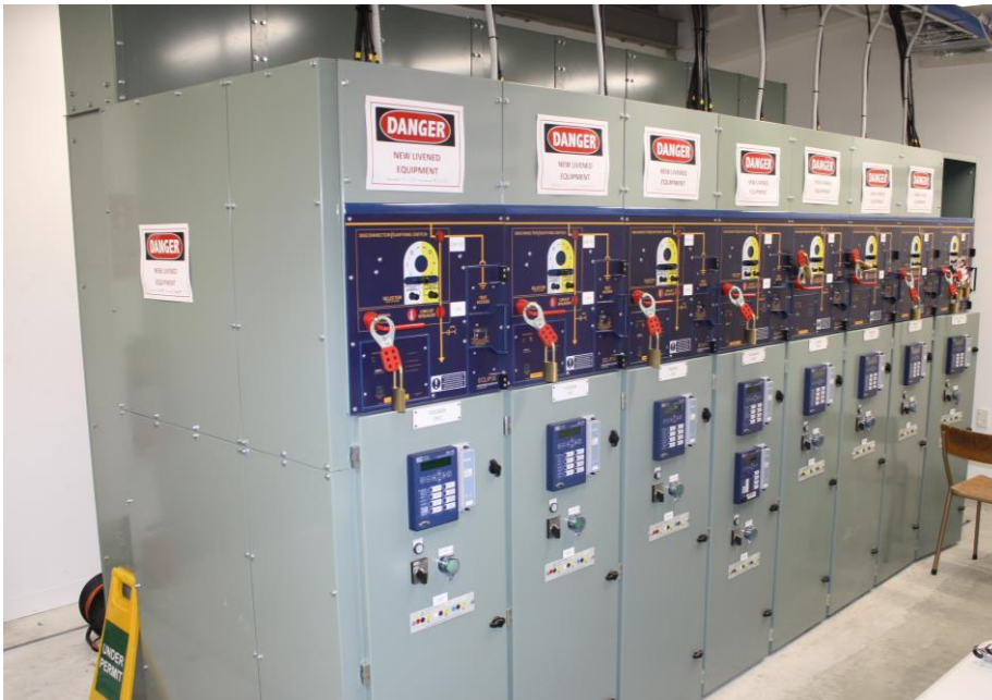
Figure 8.54: Modern 11 kV vacuum interrupter indoor switchboard at Carisbrook zone substation
