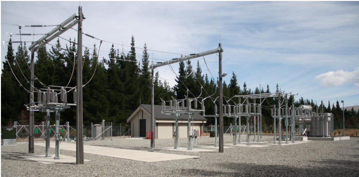
Figure 8.49: Camp Hill zone substation
