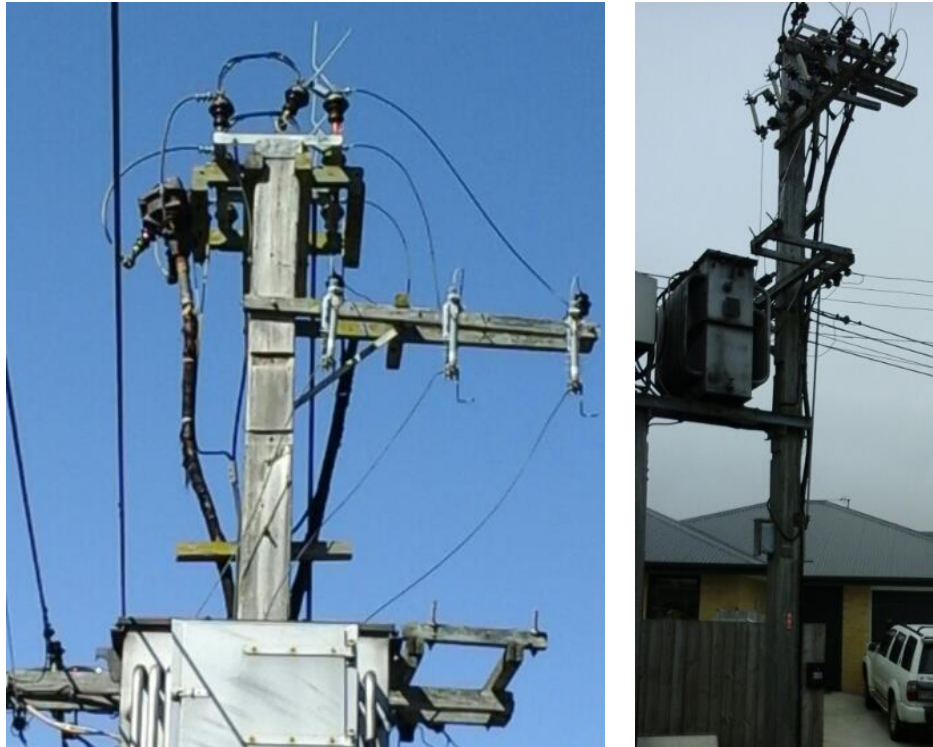
Figure 8.91: Legacy pole-and-a-half substation with an ABS and two cast iron cable terminations
