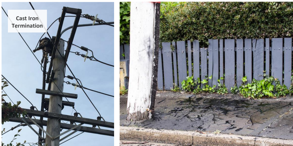
Figure 8.41: Cast iron cable termination (left) and bitumen sprayed after cast iron cable termination failure
