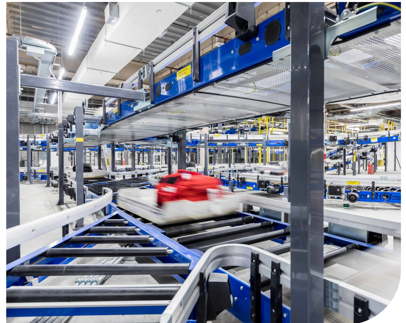
The innovative new individual carrier system uses less equipment and airport footprint than traditional baggage handling systems, and is five times faster.
