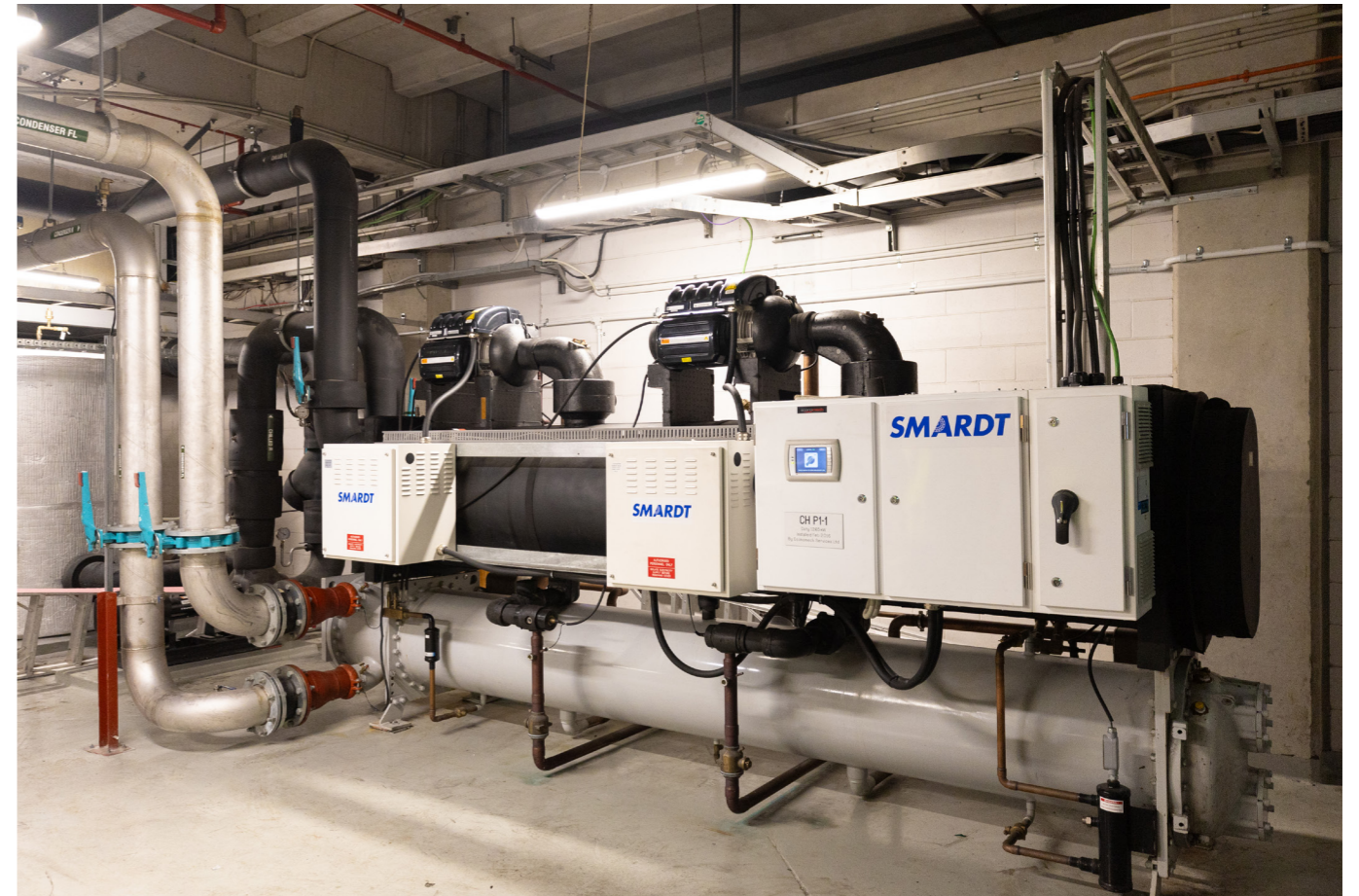
Innovative heat pump technology that warms and cools air simultaneously within the same unit is one of the first large-scale units of its type in New Zealand.
