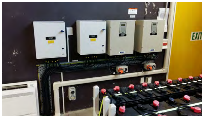
Figure 35: Battery chargers and fuse boxes, with battery banks in the foreground
