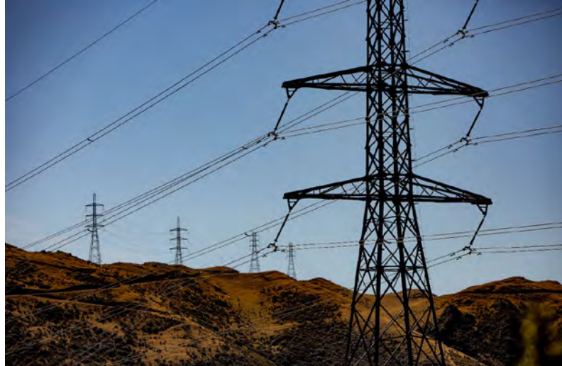
Figure 25: Transmission tower and insulators
