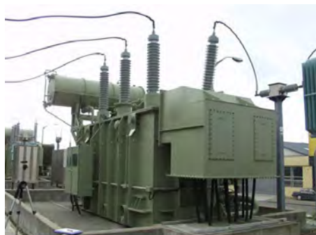
Figure 30: A typical three-phase transformer
