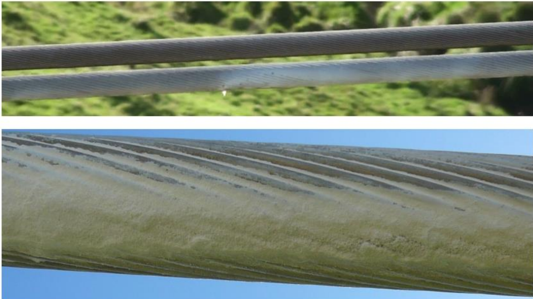
Figure 3: Conductor defect on span 54A-55A shows extent of white corrosion product on the underside of the conductor before removal from the line
