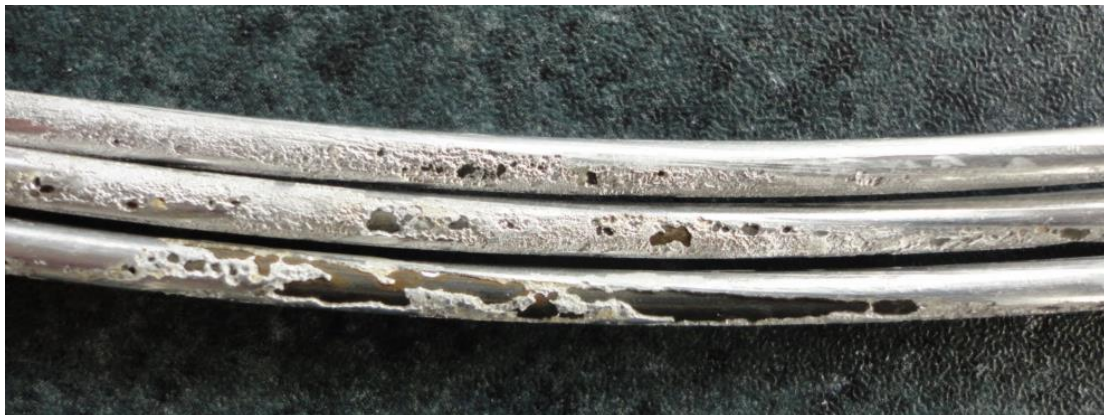
Figure 4: Exposed steel on aluminium-clad steel core wires (span 67A – 68)
