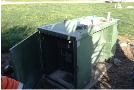
Distribution substation, LV end
