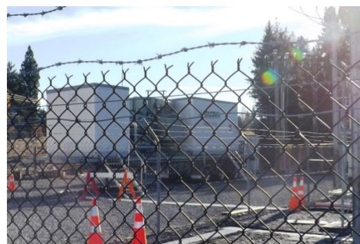
Mobile substation parked at Tekapo
