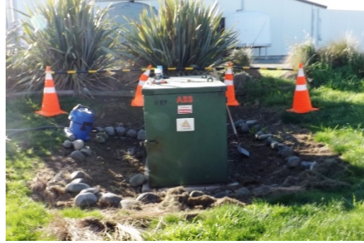
Showing ground level issue
