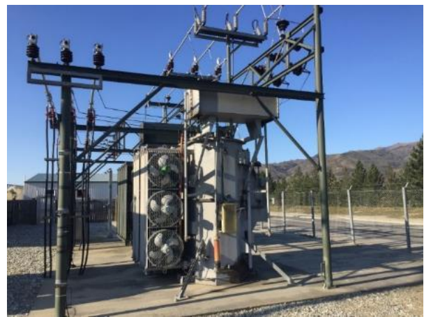
Photo 3: Cromwell ZSS – T1 & T2 adjacent to each other; no fire wall between units (impractical because of overhead bus), no oil bund; main road adjacent
