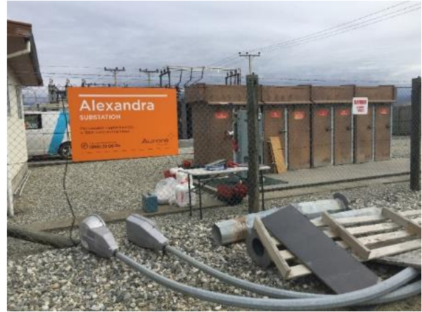
Photo 2: Alexandra ZSS – 11 kV feeder CBs; indoor ASEA HKK CBs in an outdoor enclosure; Flammable Pinex lined internally; 11 kV bus generating partial discharge
