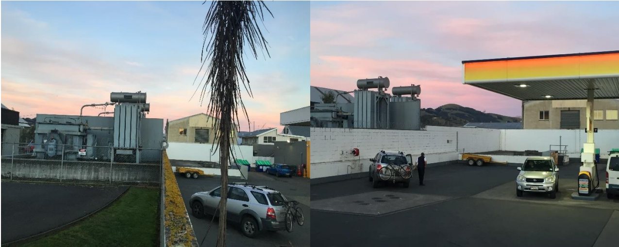
Figure 15.2 East Taieri zone substation transformer adjacent a petrol station
