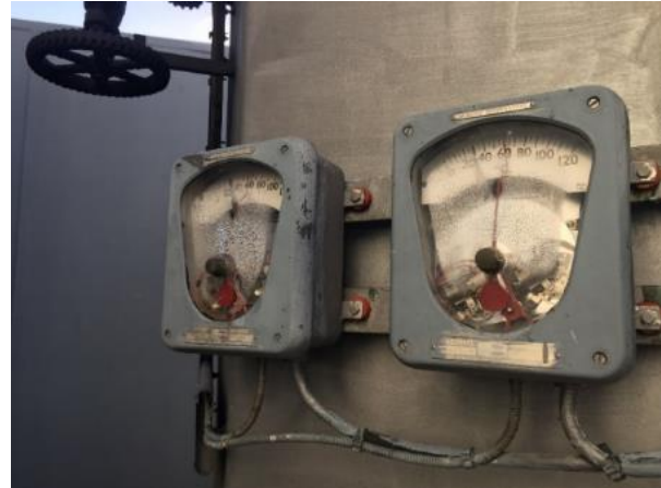
Photo 9: North City ZSS – transformer temperature relay mercury switch contacts (spurious trip risk in a seismic event)
