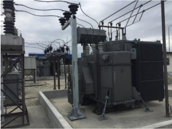
Photo 1: Alexandra ZSS – 33/11 kV T2; live 33 kV terminals approx. 2.1 m agl. ASEA CB type HPL on left
