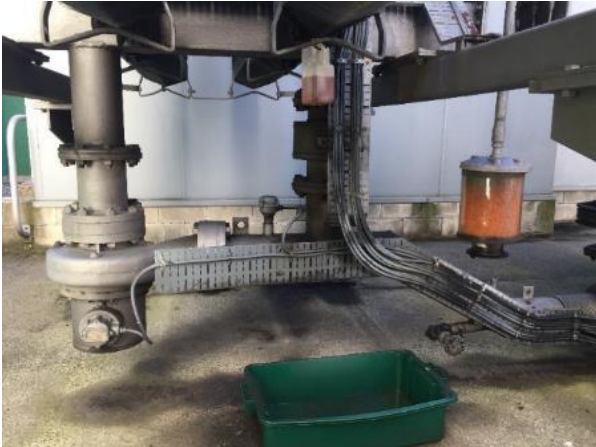
Photo 8: North City ZSS T2 – leaking radiator oil being caught in a 2L container; many radiator repairs evident
