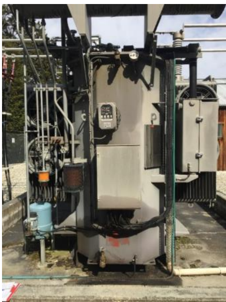
Photo 6: Fernhill ZSS T1 – oil leaking from sensor cable glands; VT fuse caps on top of transformer incorrectly fitted
