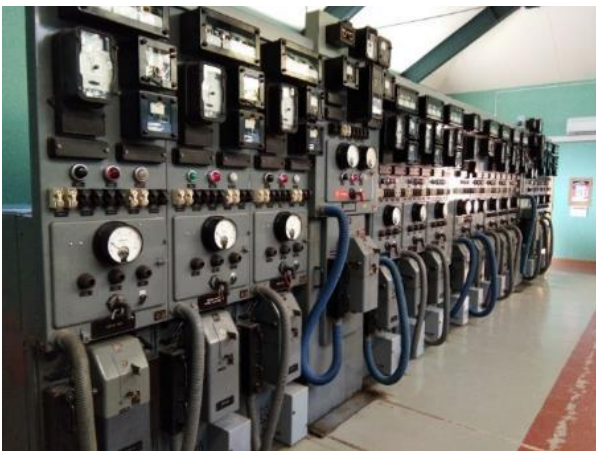
Photo 10: Halfway Bush ZSS – typical suite of 1960's 6.6 kV feeder CBs, electromechanical protection relays, bulk oil CBs
