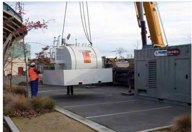
Installing large diesel generators in QEII park to provide backup power supply if needed.
