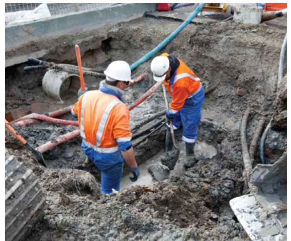
Repair crews replace damaged 11kV cables on Bexley Road. Since the earthquakes we've seen more than 1,000 cable faults on our network – more faults than we usually see in a decade.
