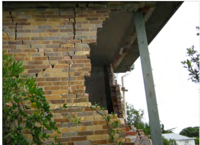
Seismic strengthening of this substation kept the roof up. This meant the substation could remain operational while repairs to the walls were undertaken. Without the strengthening this substation would undoubtedly have been damaged beyond repair.
