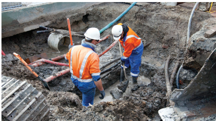
Repair crews replace damaged 11kV cables on Bexley Road. Since the earthquakes we've seen more than 1,000 cable faults on our network - more faults than we usually see in a decade.
