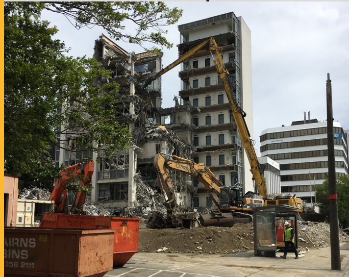
Post Kaikoura earthquake damage
