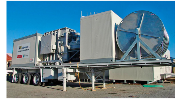
Spare mobile substation to speed up restoration
