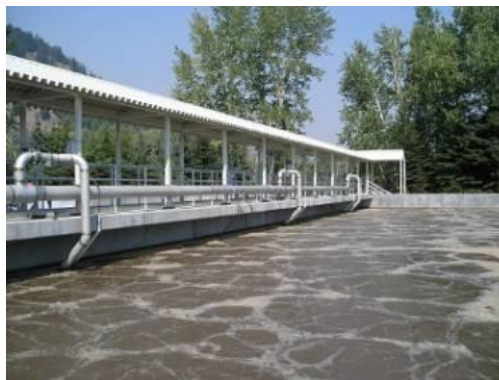
Fig 10: aerating water using a blower
