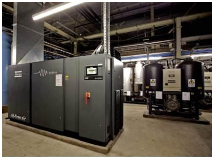
Fig 7: stationary compressor installation
