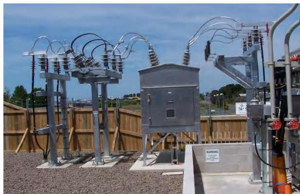
Figure 18.9: Typical outdoor 33kV switchgear bay
