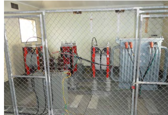
Figure 18.16: Load control injection plant
