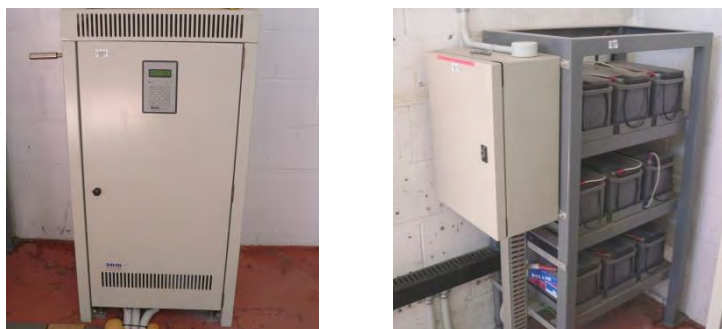
Figure 21.6: DC charger and battery bank
