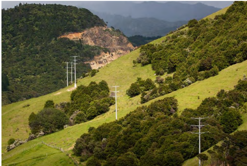
Figure 16.1: 66kV subtransmission overhead line in the Coromandel
