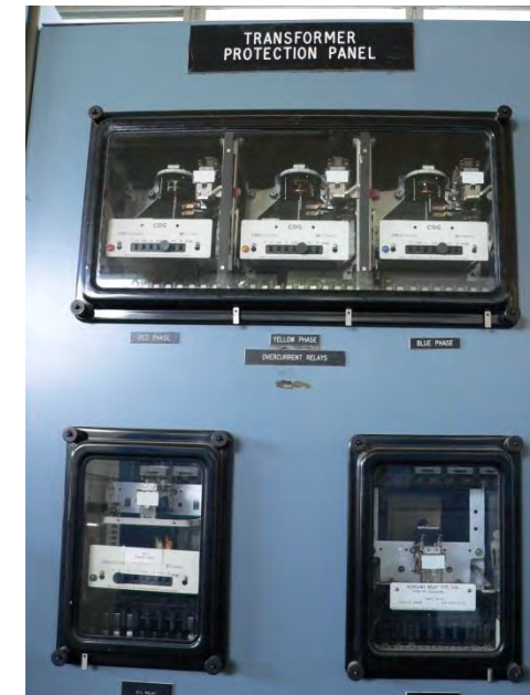
Figure 21.3: Electromechanical relays providing transformer protection
