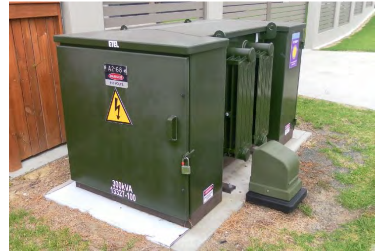
Figure 19.6: 300 kVA ground mounted transformer
