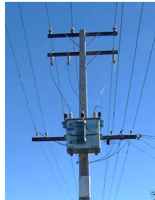
Figure 19.1: 100kVA pole mounted transformer
