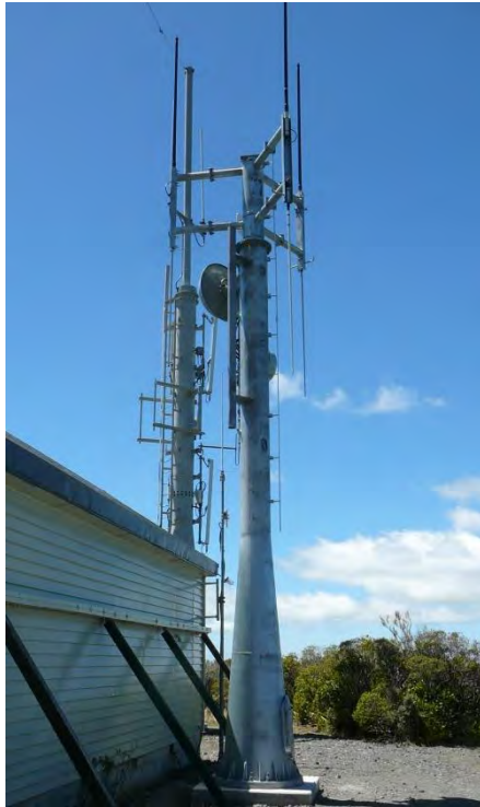
Figure 21.2: Communications mast with associated radio antennae
