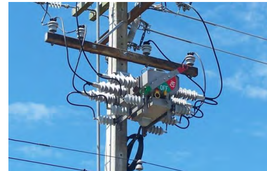
Figure 20.15: A pole mounted recloser
