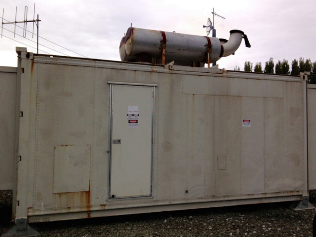
Figure 30 - 1 MW diesel genset at Matawhero
