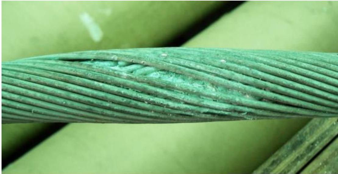
Figure 4 - Conductor bulge due to grease holidays (CPK-WIL B Span 14-15)
