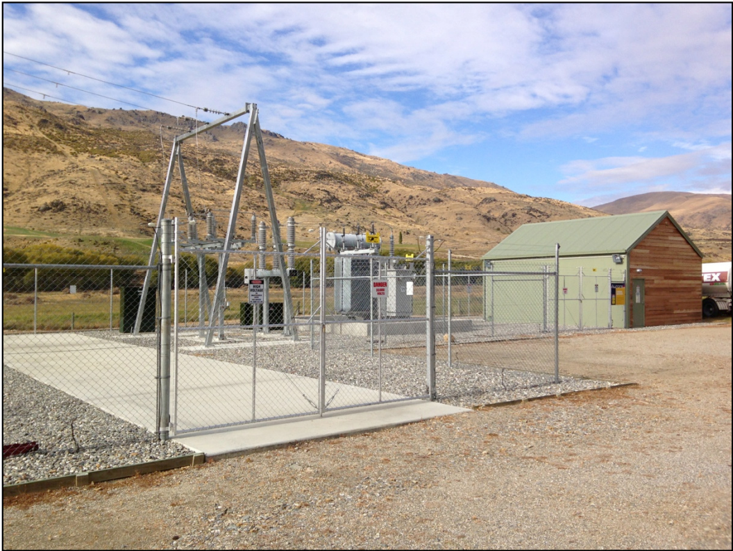
Figure 6 - Cardrona zone substation and 66 kV line
