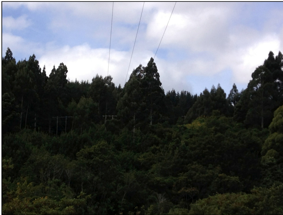
Figure 7 - Severe vegetation issues – Otago Peninsular 33 kV lines
