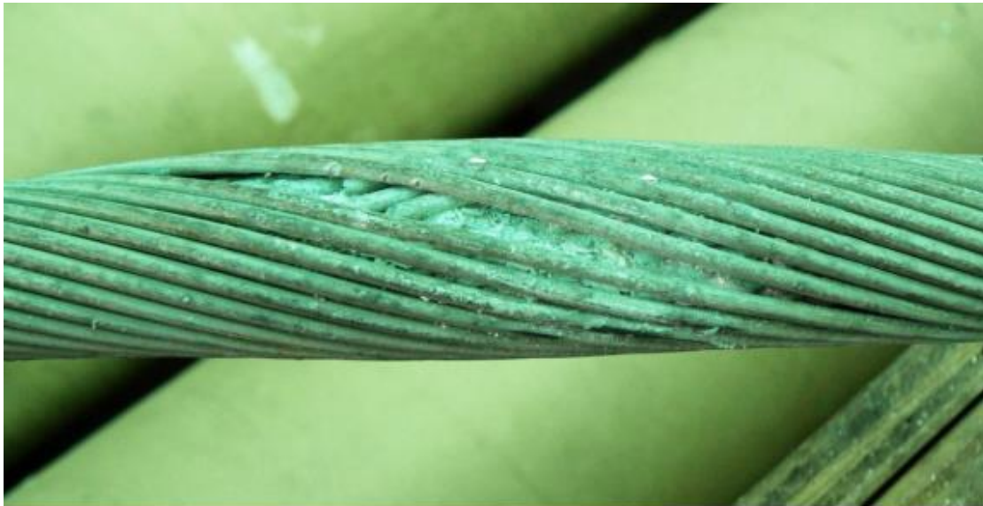
Figure 2 - Conductor bulge due to grease holidays (CPK-WIL B Span 14-15)
