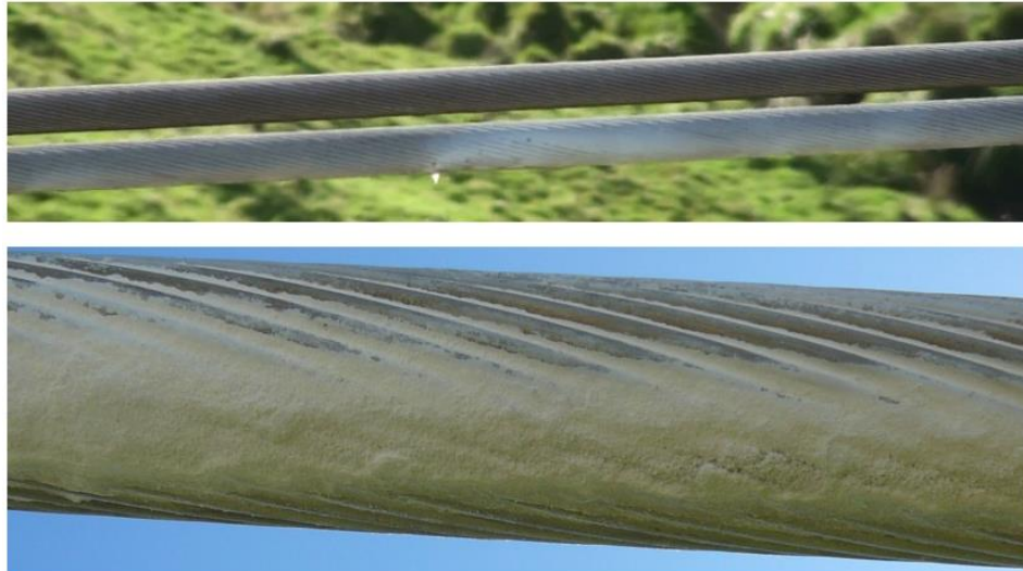
Figure 5: Conductor defect on span 54A-55A shows extent of white corrosion product on the underside of the conductor before removal from the line
