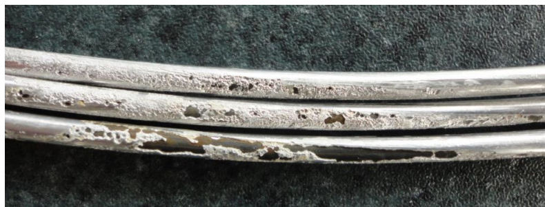
Figure 6: Exposed steel on aluminium-clad steel core wires (span 67A – 68)
