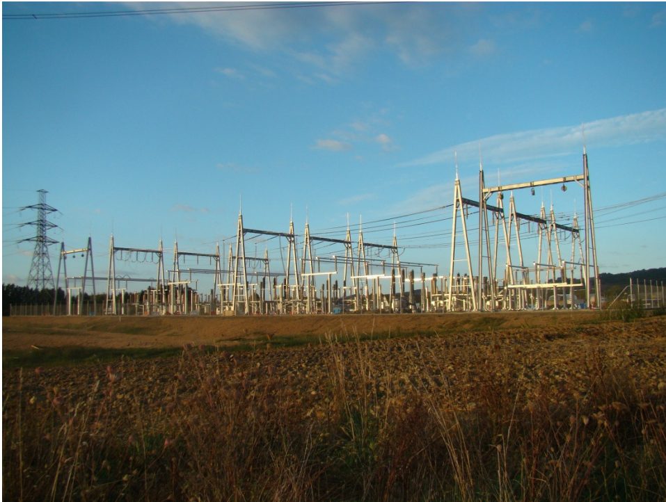
Figure 10-1: Drury switching station
