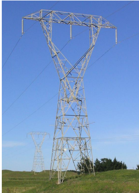
Figure 2 - Bunnythorpe–Haywards A and B 220 kV single circuit 'flat top' towers, typical of most of the line route
